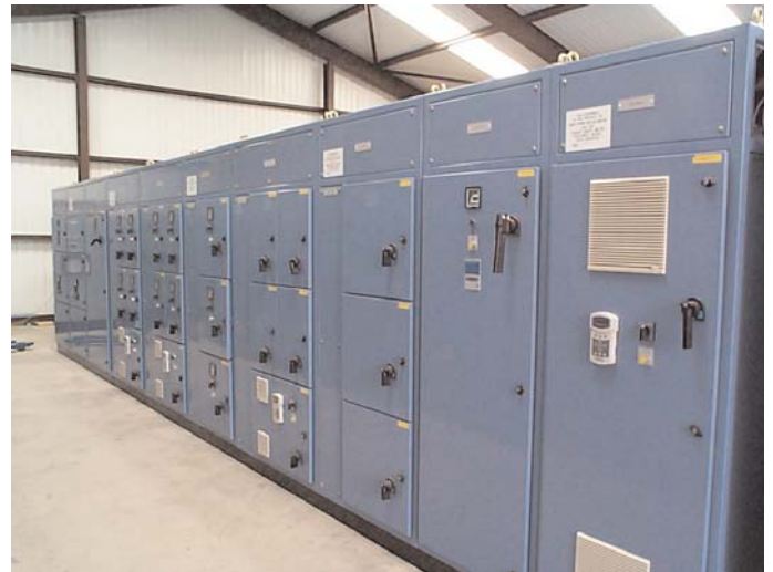
A typical panel from Lloyd Morris Electrical
